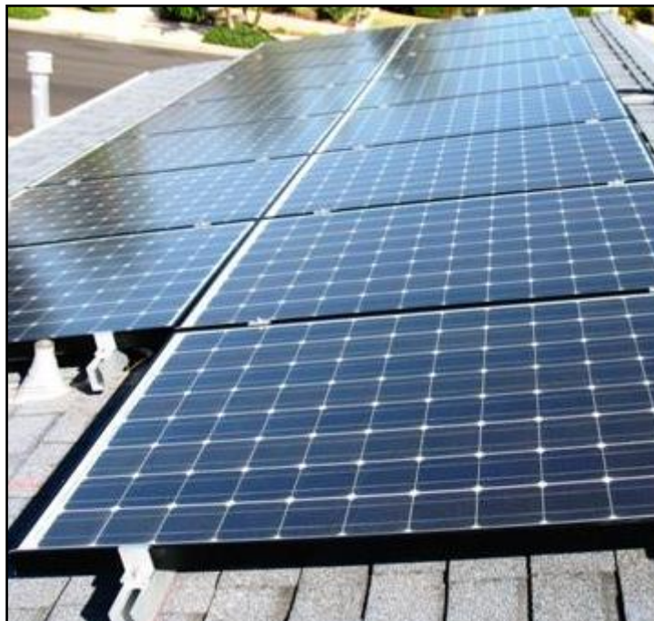
Photograph 1: Typical Roof Mounted PV Installation Source: AECOM Technology Corporation
